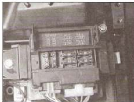
5.1a On EX models the fusebox is located on the junction box ...
