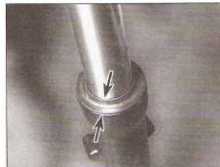
17.3 Check above and below the fork seals (arrowed) for signs of oil leakage
