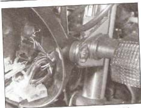
9.7a Remove the throughbolt and nut from each side of the headlight . . .
