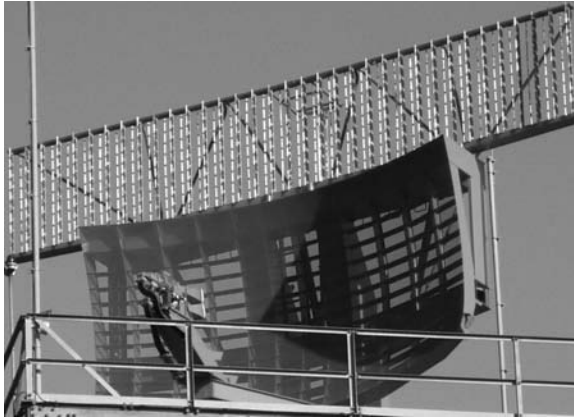
FIGURE 43-10 Open-array SSR antenna. The ladder-like top section makes up the SSR directional antenna.
